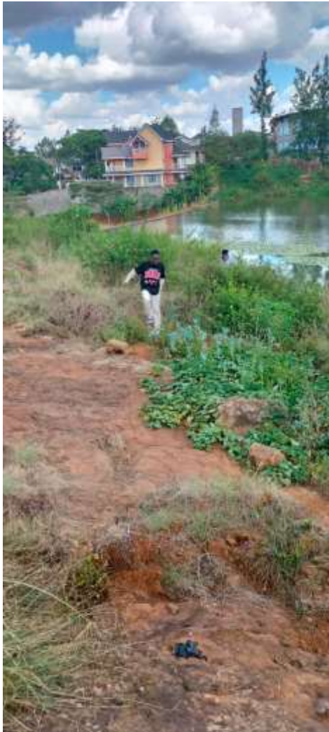
Photo: 1 Eroded left bank of Muchuki dam and top of weir in back ground
