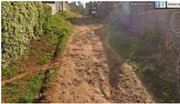
Photo: 15. Badly eroded and drained road in Michuki residential area
