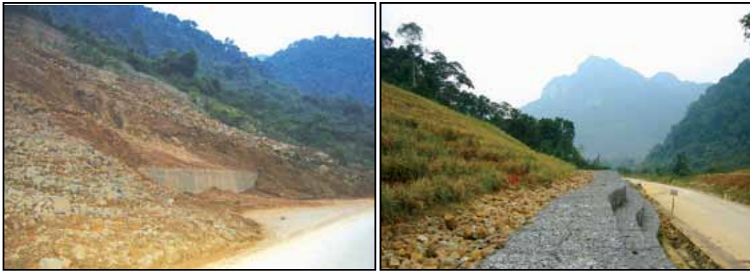
Photo 21: Da Deo Pass, Quang Binh: Left: Vegetation cover is destroyed, revealing ugly and continuous failures of cut slopes; right: Vetiver rows on top of the slope very slowly squeeze down, considerably reducing the failed mass.
