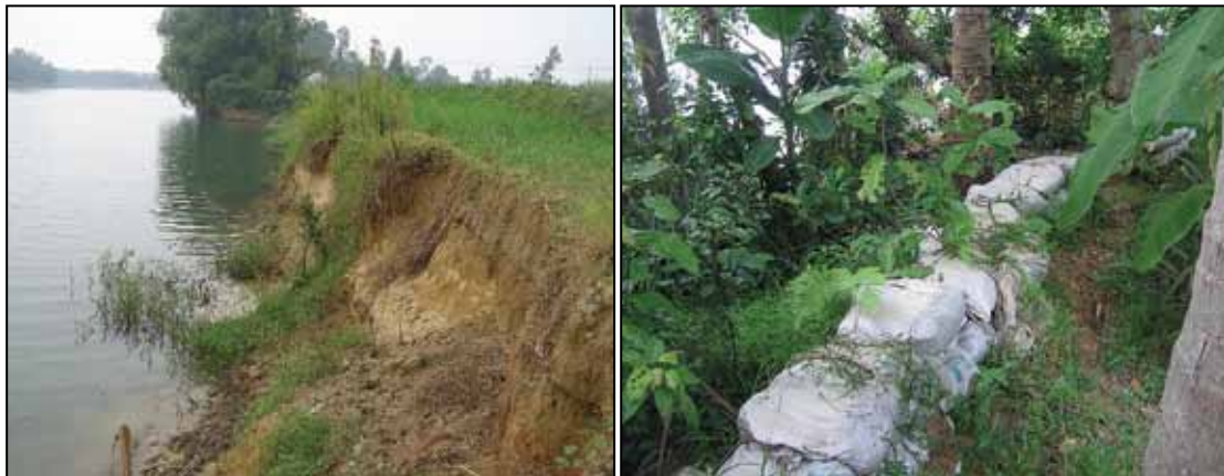
Photo 13: Left: severely eroded bank of the Tra Khuc River, at Binh Thoi Commune; right: primitive sand bag protection.
