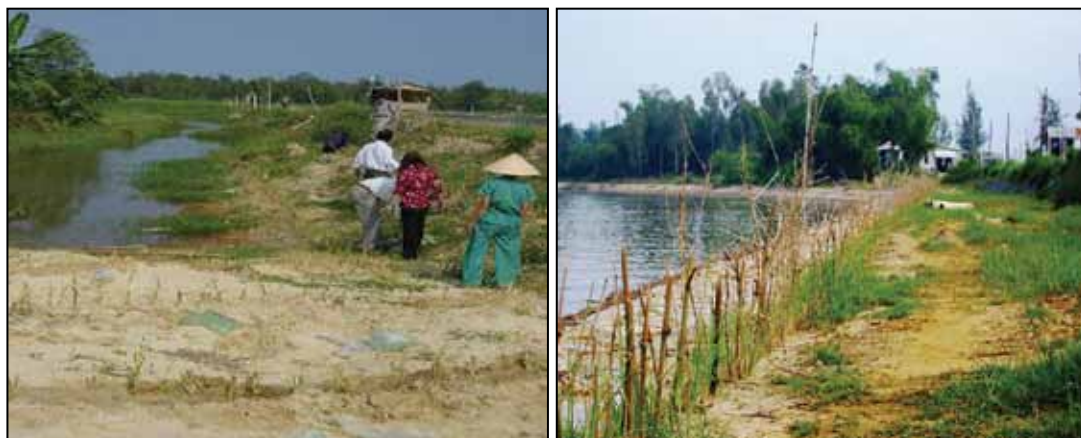
Photo 8: Left: March 2002: VS trial at the edge of a shrimp pond, where a canal drains flood water to Vinh Dien River; right: November 2002: mass planting combined with rock riprap to protect bank along Vinh Dien river.
