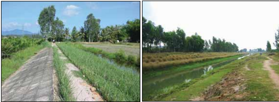
Photo 12: Upstream anti-salinity dike section with traditional concrete riprap facing the river (left) and along a section of the irrigation canal, surface erosion mars the opposite bank (right).
