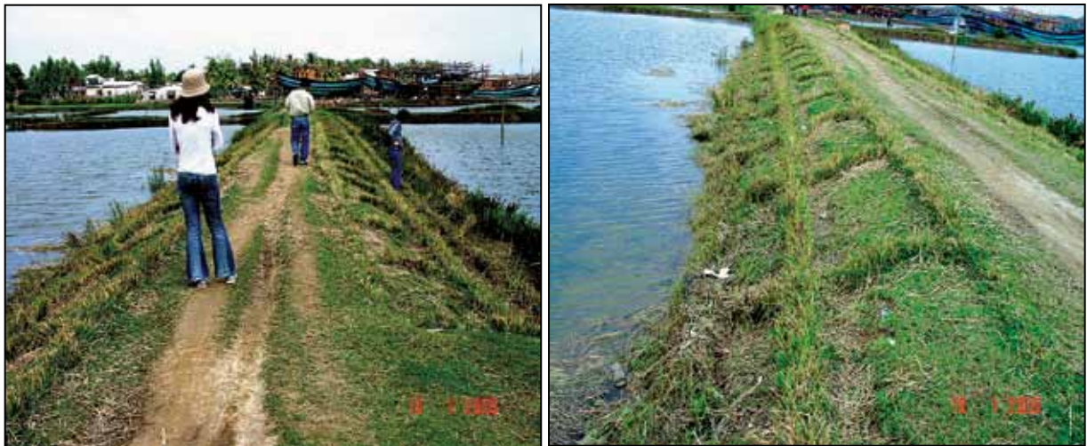
Photo 22: Vetiver, installed in a cross-hatched pattern, protects shrimp pond dikes in Quang Ngai.
