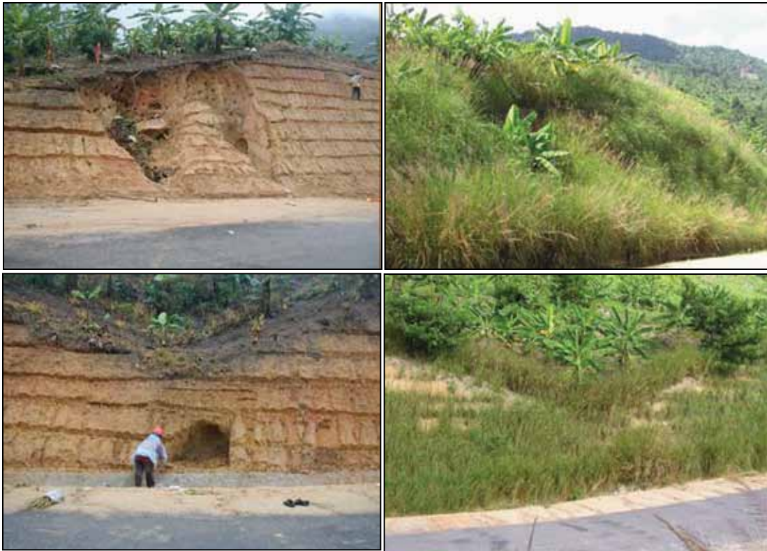
Photo 22: Pham Hong Duc Phuoc, a road protection project in Khanh Hoa province, road to Hon Ba): left two photos: severe erosion on newly built batter occurs after only a few rains; right two photos: eight months after vetiver planting: Vetiver stabilized this slope, totally stopping and preventing further erosion during the next wet season.
