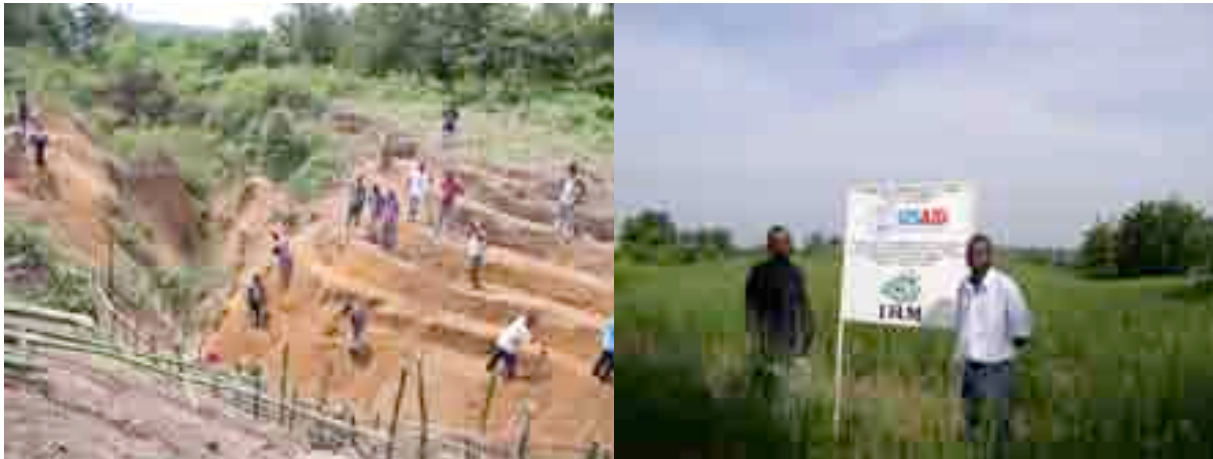
Slope preparation on the left, and the final product after 4 months on the right with the Alain Ndona (right of the sign) who worked with the community on this gully reclamation.
