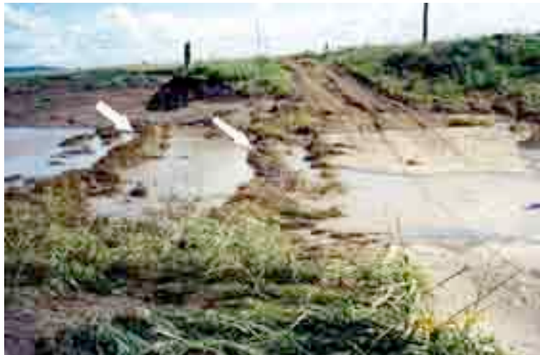
A 2 meter flow of flood water passed over this "Irish Crossing" on a farm in Australia. Vetiver hedgerows were planted upstream and adjacent to the crossing, and as a result the high velocity flood water was unable to undercut and break up the concrete (in previous floods, without vetiver protection the crossing was destroyed and had to be rebuilt. Photo by Paul Truong
