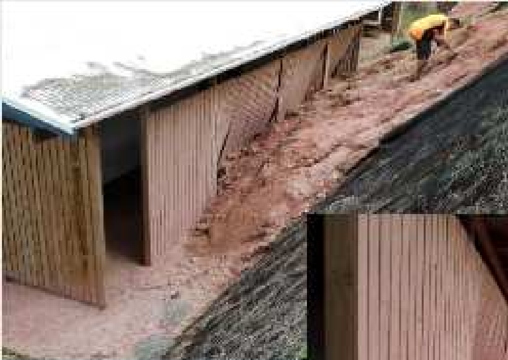
Slope slippage with damage to building
