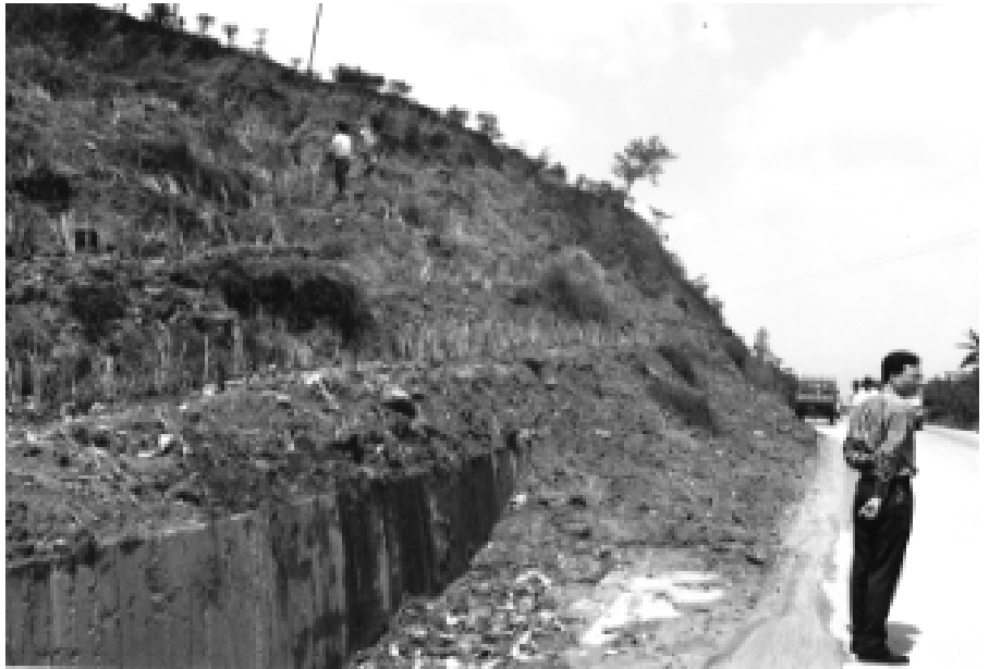
Photo 2: China. Guangdong Province. A slipping highway cut just planted to vetiver.
