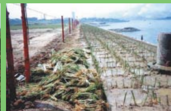
China - the embankment on the image to the left was reshaped and planted with vetiver grass hedgerows. Hedgerows were planted perpendicular to each other
