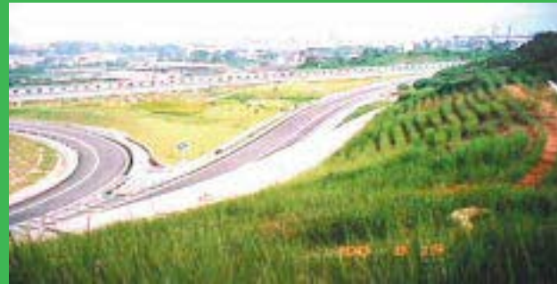
China - the same cut 12 months later. This cut was prone to massive slip. Stabilization with VS has given complete protection
