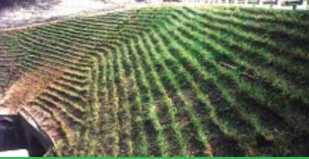
El Salvador - Highway fill section treated with VS. Applications such as this provided full protection during Hurricane Mitch
