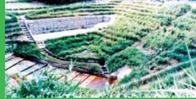
Malaysia - VS applied to major expressway through drainage system
