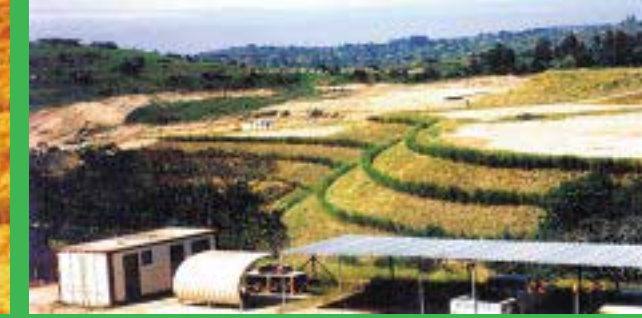
South Africa - VS applied to stabilizing a construction site. Indigenous species were seeded between vetiver hedgerows
