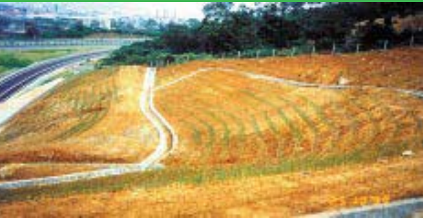
China - a highway cut just planted to vetiver. The soils are very acid and prone to slippage. High levels of fertilizer assure good growth
