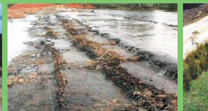
Australia - this causeway was regularly damaged by flooding. Gabions were often washed out
