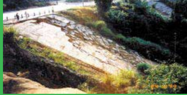
China - engineering solutions are expensive and often break down when tied to fragile soils, particularly under high rainfall conditions
