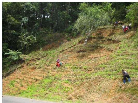
Figure 12 : Vetiver system was applied for stabilizing and stopping soil movement on highway slope ( Route No.1249 ).
