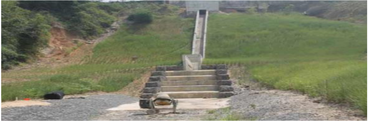
Figure 4: Reclaimed Atakpa site in Cross River State using VST and Reinforced Concrete structure (www.newmap.gov.ng)
