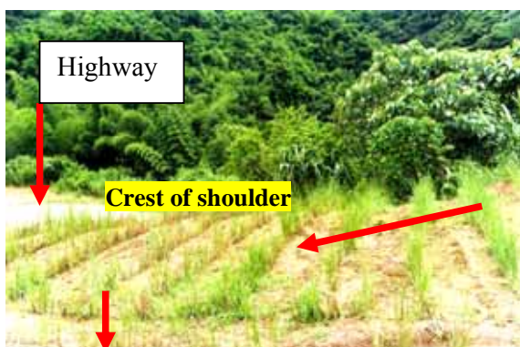
Figure 5 : Vetiver planting at steep gradient of highway shoulder to slow down runoff longitudinal.
