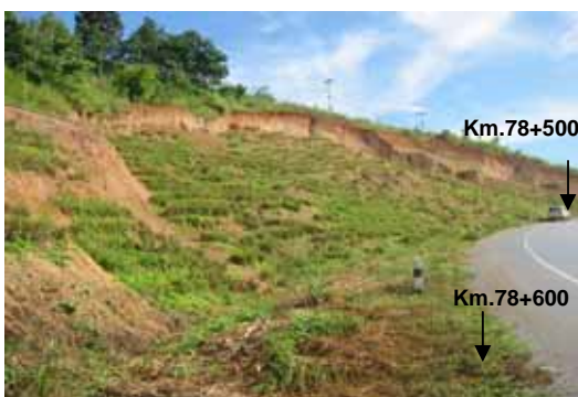
Figure 11 : Highway cut slope was stabilized with vetiver for stopping the earthflows on Highway Route No.107 (in 2007).
