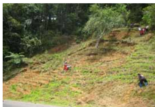
Figure 12 : Vetiver system was applied for stabilizing and stopping soil movement on highway slope (Route No.1249 ).
