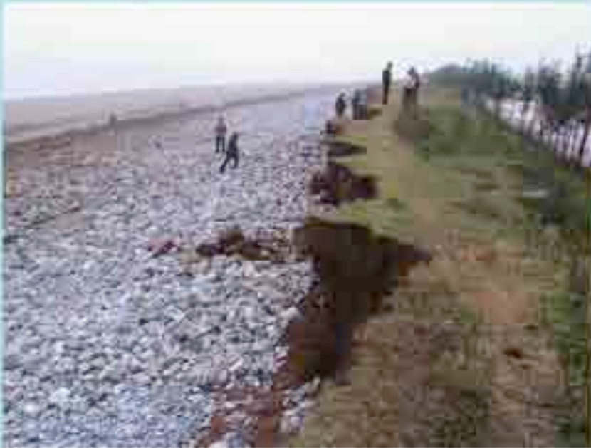
Typical erosion on the sea facing batter of an old dike along the coastal zone facing Ha Long Bay. Note the collapse of the gabion/rock basket armour
