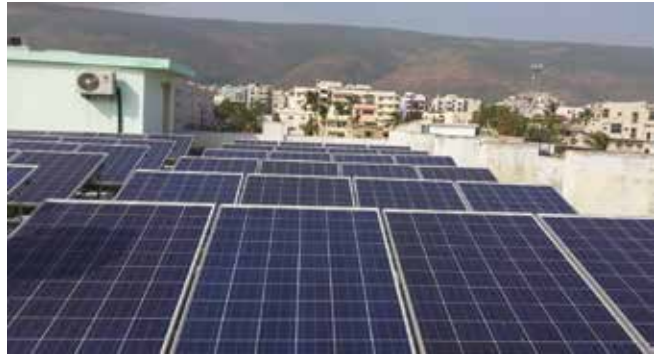
Figure 31: Rooftop Solar Panels in Andhra Pradesh
