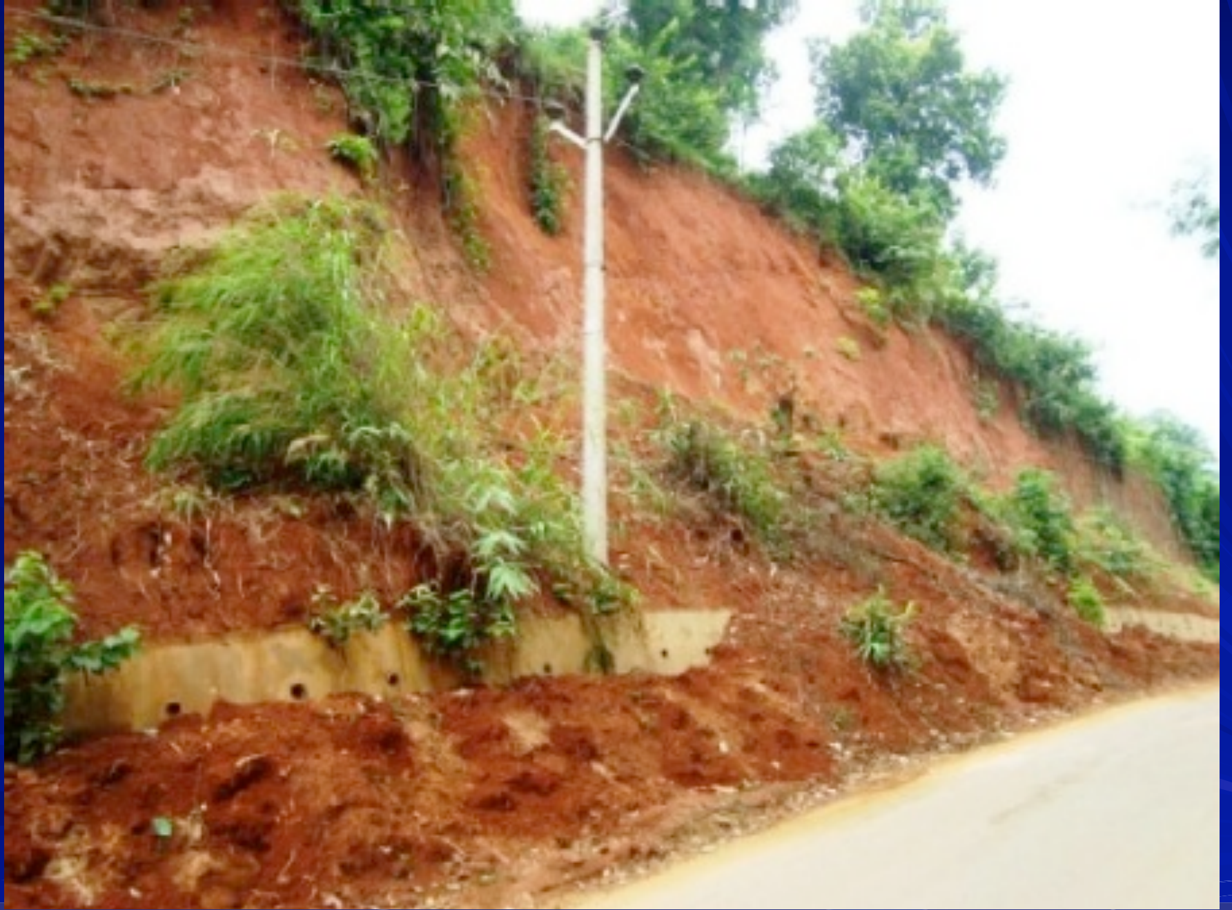
Severe land slide on Noonmati- Kharghuli Road
