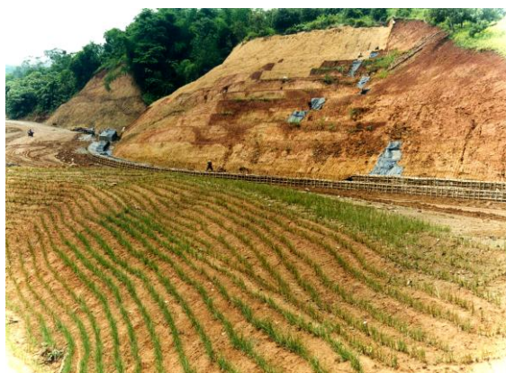
Figure 7: Vetiver were planted as pioneer plant on barren land for highway construction project.
