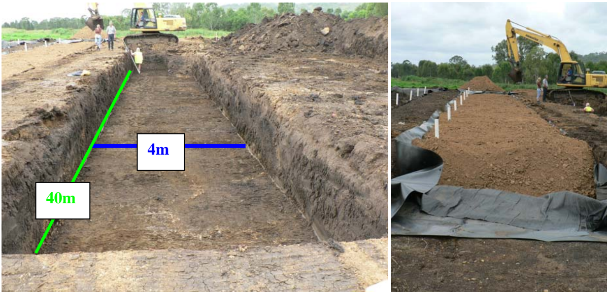
Photo 1: Box cut with 1% gradient (left), and lined with High Density Polyethylene sheet and filled with soil (right)
