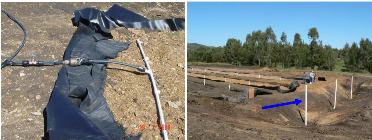
Photo 2: Inlet system (left), and outlet system (right)
