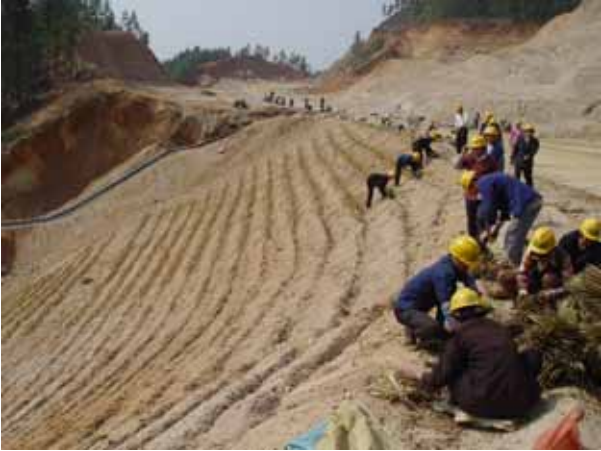
Fig. 17 Vetiver was being planted on contours of the above highway in the beginning of 2003
