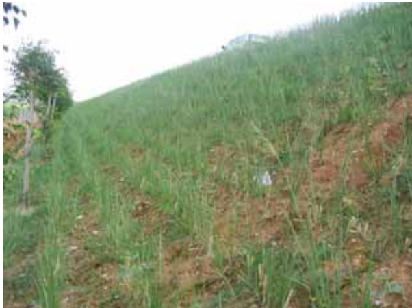
Fig. 14 A vetiver project in the section of the highway one month after planting vetiver
