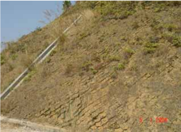
Fig. 21 A failed project of planting grass in lattices set on a slope of the reservoir conducted several years ago
