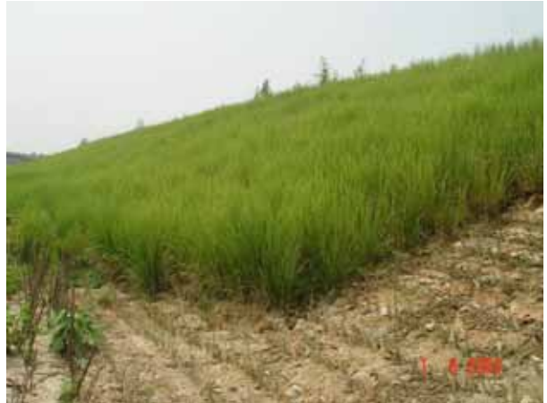
Fig. 15 Another vetiver project in the same section three months after planting vetiver. Please note, vetiver cultivar in here is Karnataka
