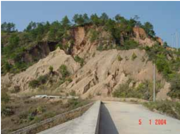
Fig. 22 A slope of the reservoir assuming severe collapse, which would be reined with the vetiver eco-engineering
