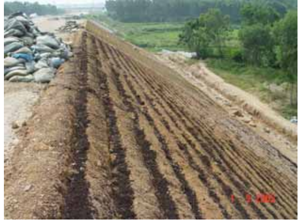
Fig. 13 A section of slope on the Zhangjiang section of Zhangjiang-Chongqing highway that is ready, dug up and manured, to be planted with vetiver
