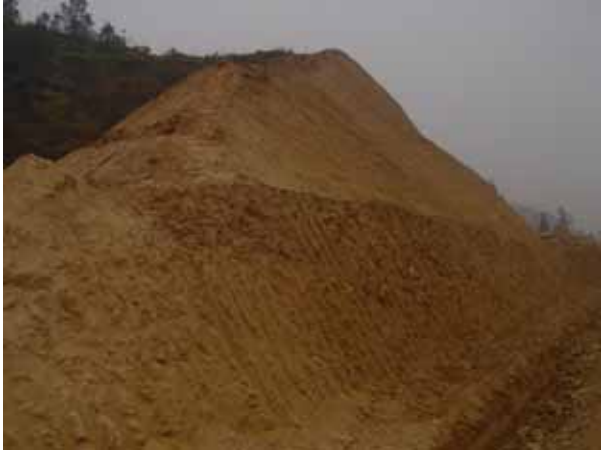
Fig. 16 A section of up-slope along the Ganzhou-Chongyi Highway that was just dug up
