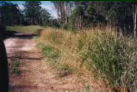
Before the fire, this 3 year old vetiver hedge planted to stabilise a railway line in Queensland, Australia
