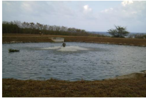
Fig. 2: At the Inarajan sewage treatment plant each cell is aerated by floating mechanical surface aerators running daily for 24 hours.
